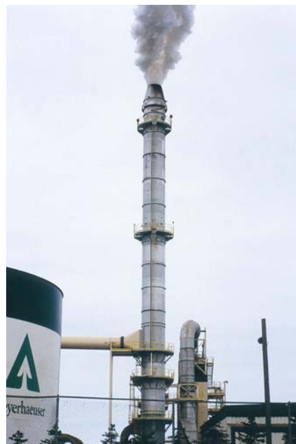
Galvanized safety platforms on stainless steel discharge stacks at Weyerhaeuser
